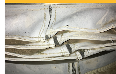
PROBLEM: DEGRADED BELLOWS
