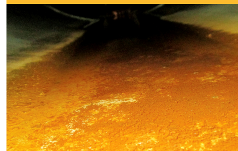
PROBLEM: WATER INTRUSION
