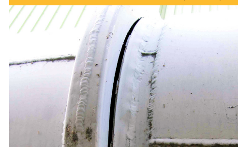
PROBLEM: CRACKED BELLOWS (METAL)
