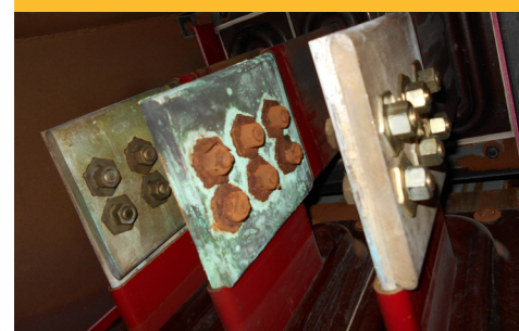
PROBLEM: DIRT/LACK OF SILVER PLATING
