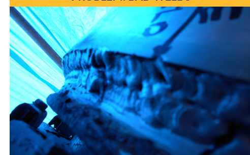
PROBLEM: BAD WELDS
